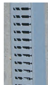
SLOTTED CABLE DUCT
